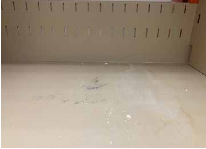
Fibers and plaster are visible on the bottom shelf of the compact shelving.
